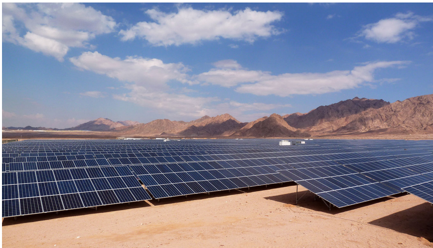
Figure 15: PV system using monofacial panels implemented at a fixed tilt (Ramboll, 2022)
