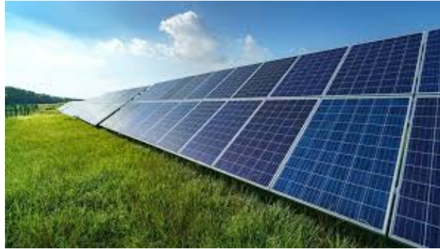
Figure 36: Stacked PV panels (Linquip Team, 2021)
